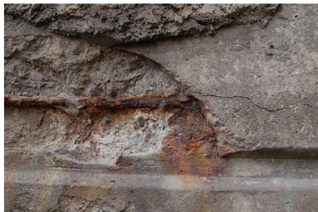
Figure 13. Concrete deteriorated from corrosion of the steel reinforcement (theconstructor.org)
