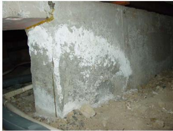
Figure 9. Concrete deteriorated from external sulfate attack (theconstructor.org)
