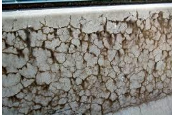
Figure 11. Concrete deteriorated from alkali silica reactions (theconstructor.org)
