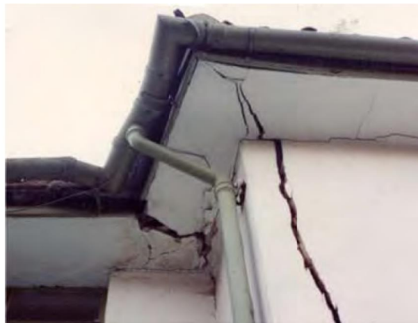
Figure 1. Building damage due to end lift (Jones (2011))
