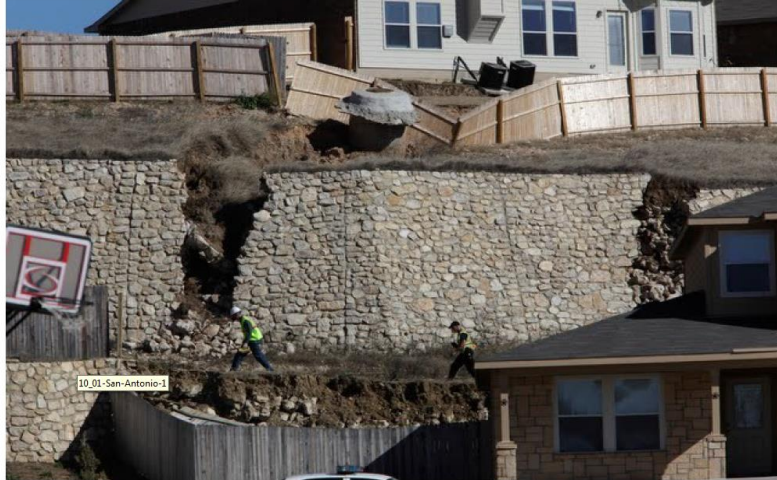
Figure 2. Retaining wall collapse due to lateral swelling pressure (Dave (2010))
