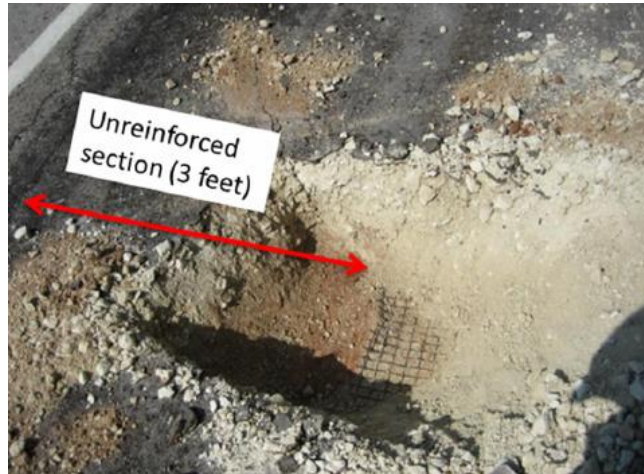
Figure 15. Incomplete coverage of the shoulder section by the geogrid layer induced a longitudinal crack, (Zornberg and Gupta (2009))
